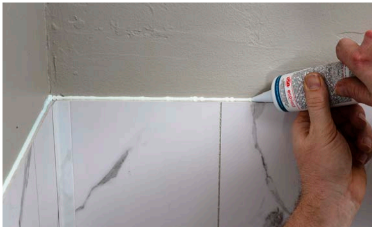
Apply sealant to top edges of all the panels for a watertight seal.
